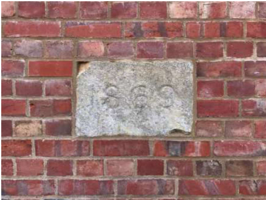
Figure 93: Date-stone of 1869 reset into gable end of south-west portion of church building (photograph taken 17 th January 2020).
